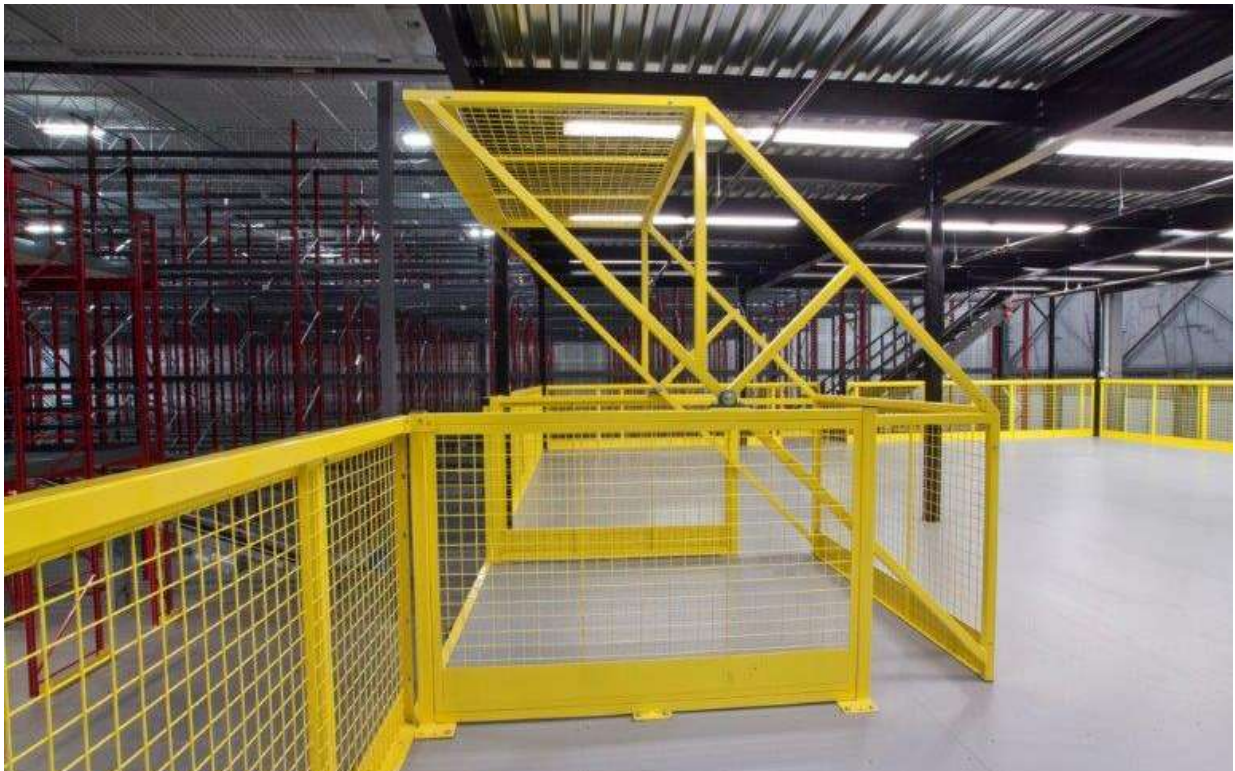
Teeter Gate Installed (Open Position)
